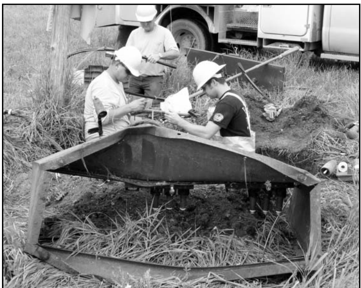
This three phase underground junction box was hit and damaged by farm equipment. Cooperative line personnel work to repair and/or splice many pieces of underground cable. The junction box had to be replaced.
